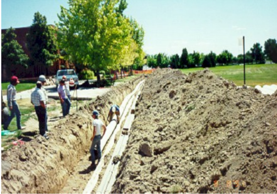
Figure 4 - The College of Southern Idaho converted much of the campus' heating system to geothermal in the 1980s. Photo credit - Don Buetner, College of Southern Idaho.
