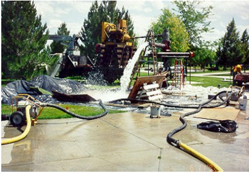
Figure 3 - The College of Southern Idaho had two geothermal wells drilled on campus. Photo courtesy of Don Buetner, College of Southern Idaho.
