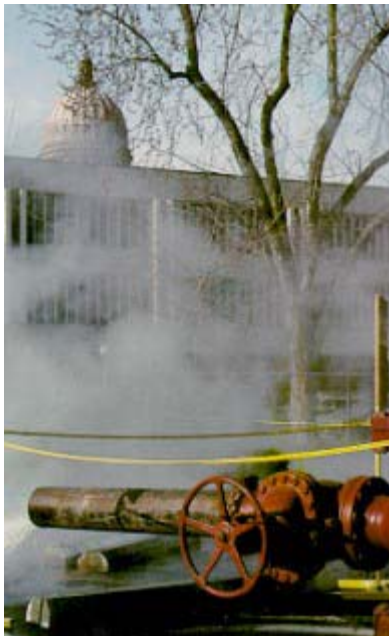
Figure 5 - Idaho has the only state capitol building in the U.S. that is heated by geothermal water.
